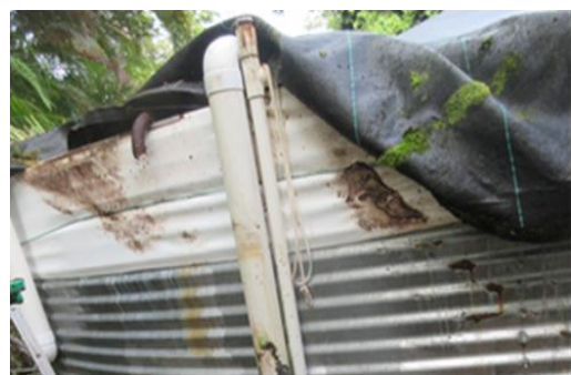
Figure13. Rainwater storage catchment
